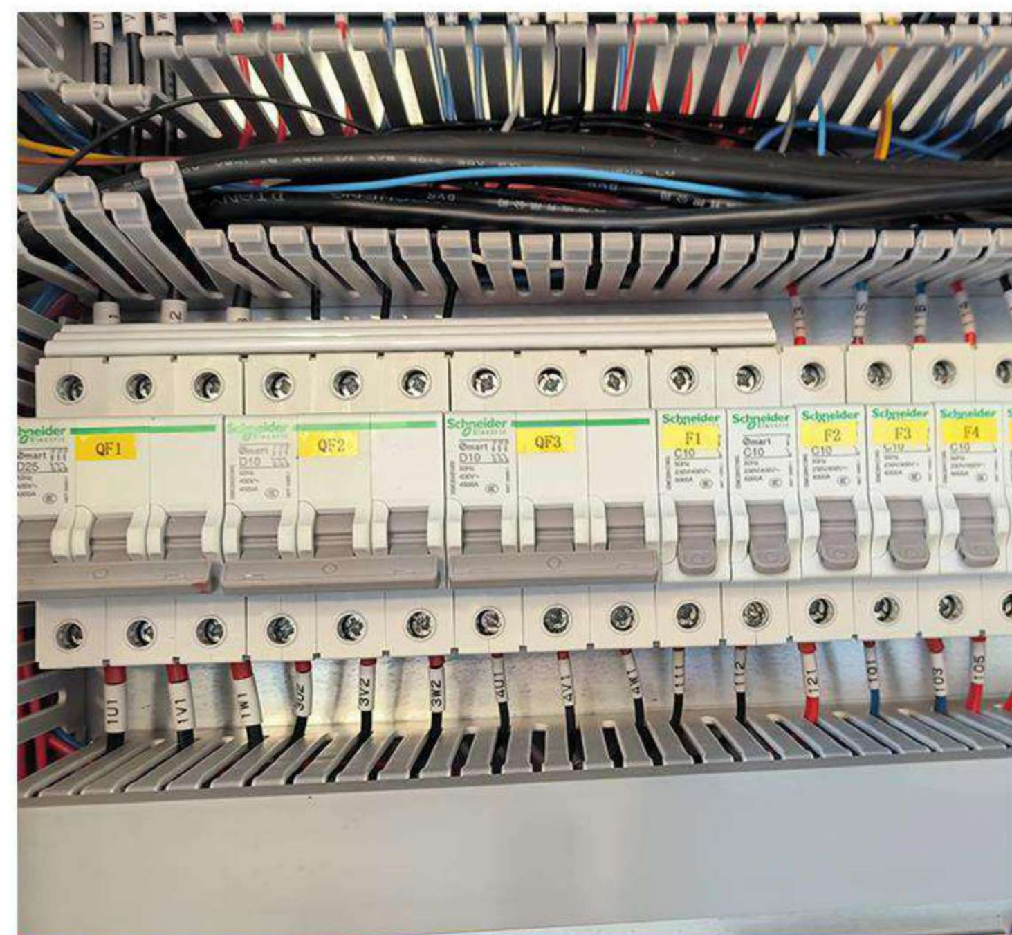
Schneider electrical components
